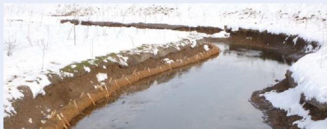
Winter view of staked coir logs for bank stabilization and coir mat on face to assist in sloughing. Photo from the Parson's Geddes Brook Onondaga - Wetlands Project
