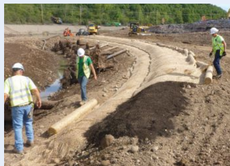
Sloughing solution utilizing straw/wool matting. Photo from the Parson's Nine Mile Creek Project
