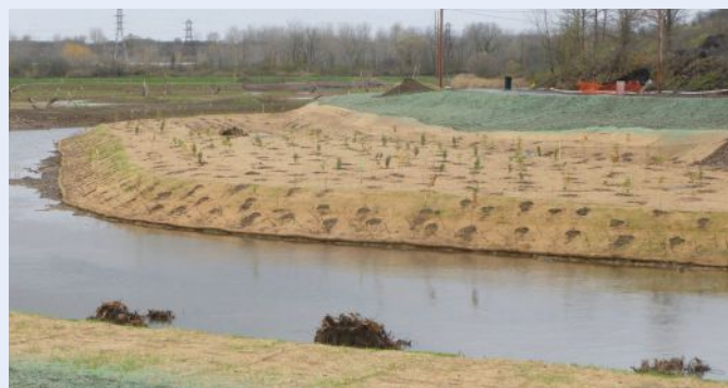
Revegetation of stream bank utilizing coir matting and living stakes at remediation site. Photo from the Parson's Nine Mile Creek Project
