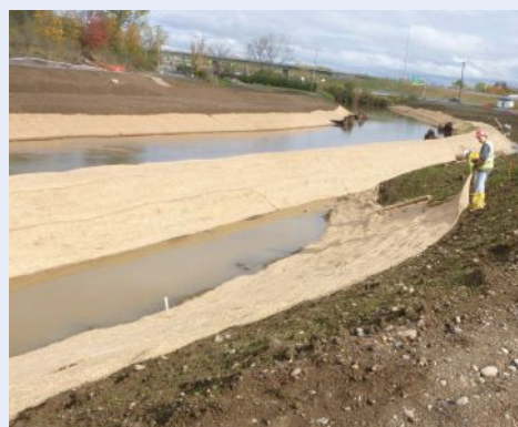
Stream bank stabilization utilizing straw/wool matting. Photo from the Parson's Nine Mile Creek Project
