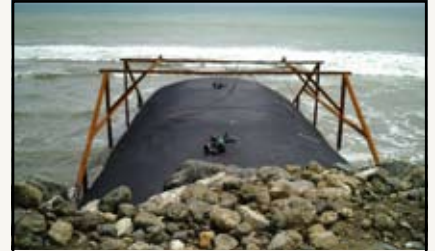
Geotube system being held in place by steel frame as it is filled.
