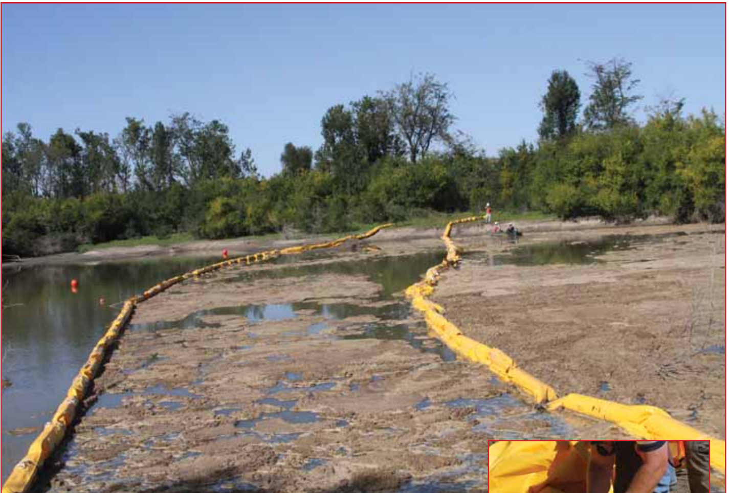
Above: Silt curtains installed parallel between the Historic Blue Hole and the scour hole. Inset: Sections of silt curtain being joined together. Images courtesy of Granite Environmental, Inc.
